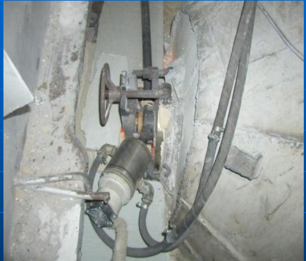
Mounted vibratory system
